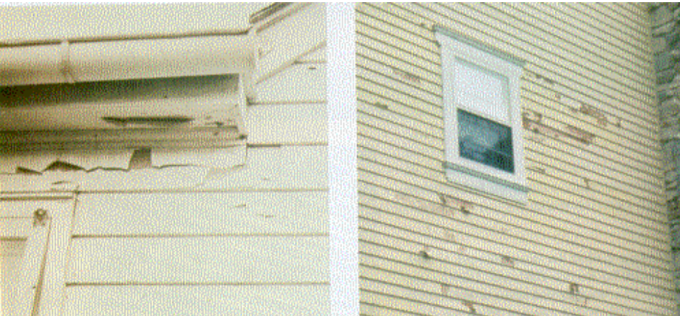
Excess moisture causes peeling paint. Leaking gutters and roofs, ice dams and inadequate overhangs are some of the typical causes of peeling paint.
